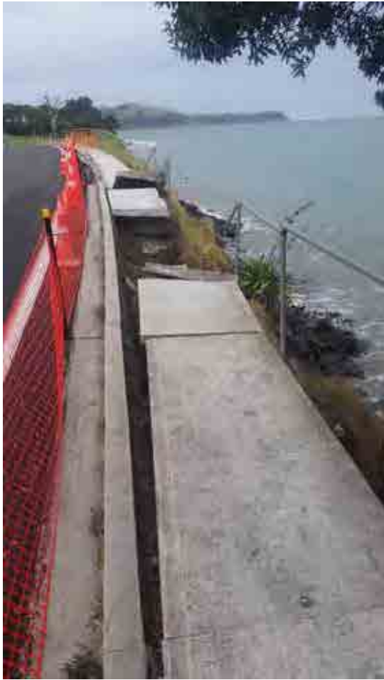
Opononi new footpath damaged from May 22/23 storm event
