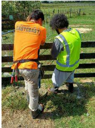
Wai Fencing students get their knots and ties right before constructing a new fence.
